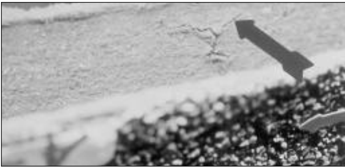
Photo 7. Close-up on bottom side of Tab A-5 of half-panel designation CO-WFB-D-7 at impact site. Note multi-line fractures radiating from common point.
