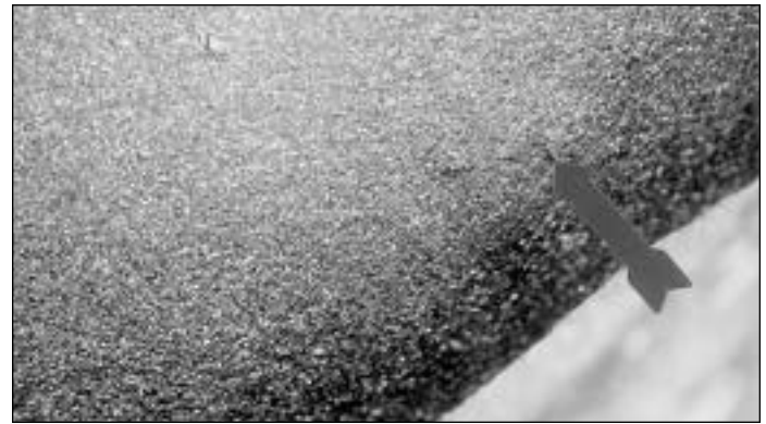
Photo 5. Close-up on bottom side of D-7 of half-panel designation CO-TS-D-7 at impact site. Note single-line fracture pattern weathered 4 years 4 months.
