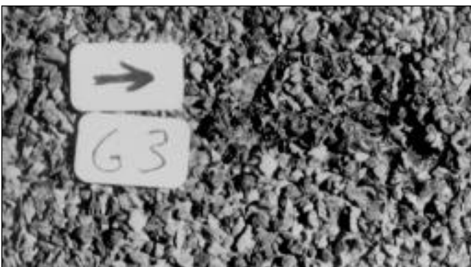
Photo 9. Close-up of Tab G-3, half-panel designation CO-FS-D-0 at 14 years 11 months weathering exposure. Note impact-caused fracture.
