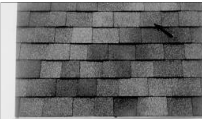
Photo D1. View of test panel at Year 0. Note D-10 at arrow.
